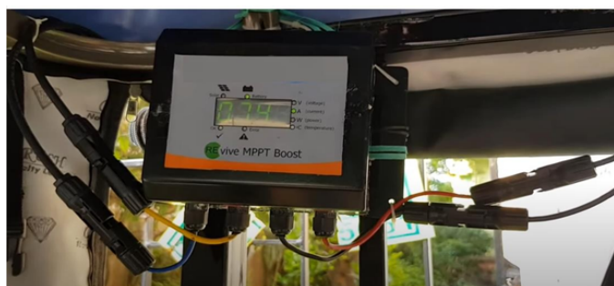
Fig 21. The Charge controller inside the solar Tom Tom
