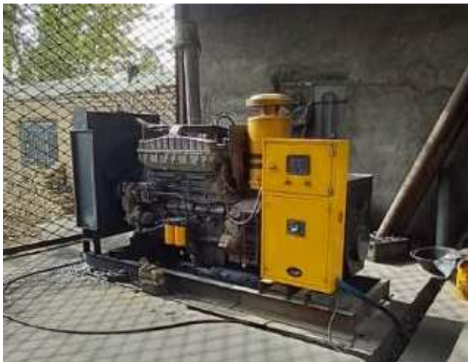
Figure 3: Primary diesel generator which is used in this site
