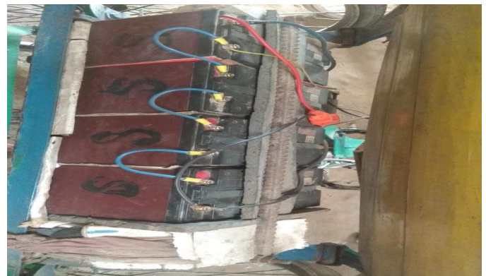
Fig 7. Most electric vehicles in the country use four batteries connected in series.
