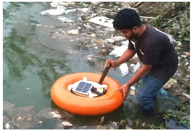
Fig. 7. Prototype installation in the canal
